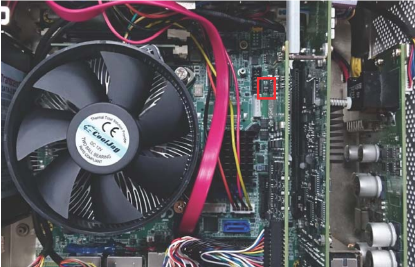
Figure 1-12: SWS1M1 Switch Location
